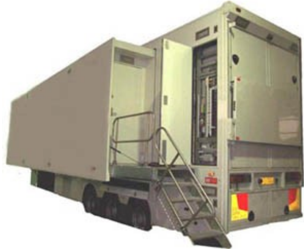
Rear view with entrance into Engineering Section and the expanding side section. Main switch board door is open
