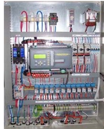
Control Panel back plate
