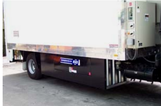
Close-up of the acoustically enclosed diesel generator and main control cubicle including weatherproof DDC access point.
