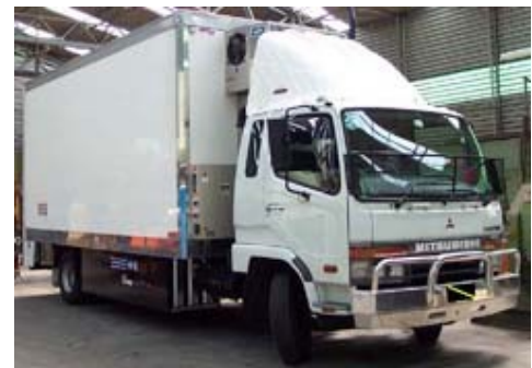
Vehicle showing under-slung diesel generator, main control panel on the front wall and the external stainless steel condensing unit on the high front wall.
