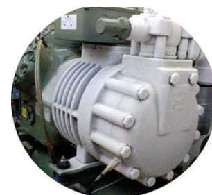
-30°C Compressor Operation during commissioning
