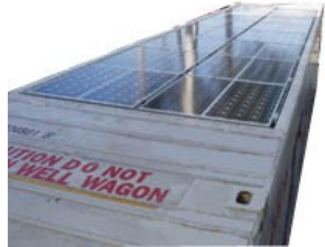
Roof mounted Solar Array
